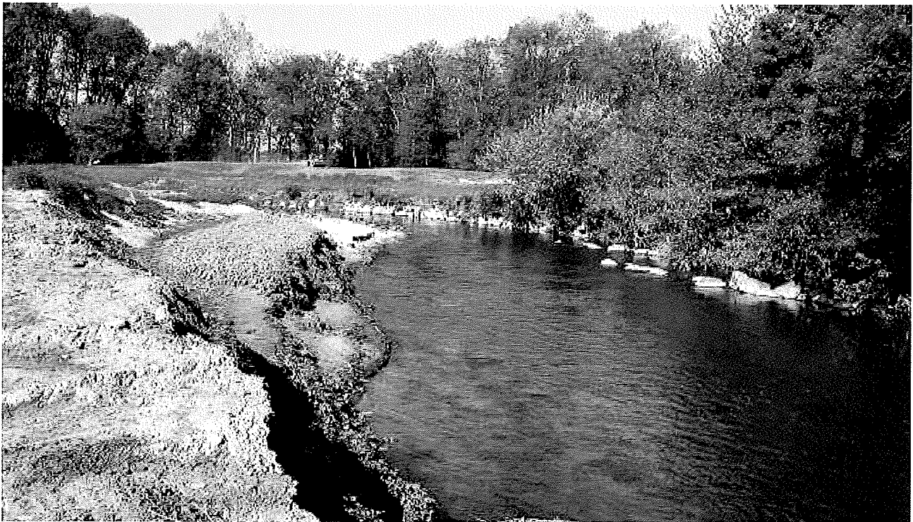
Photograph 6 – Site 4: 12 th Fairway Bank Erosion
